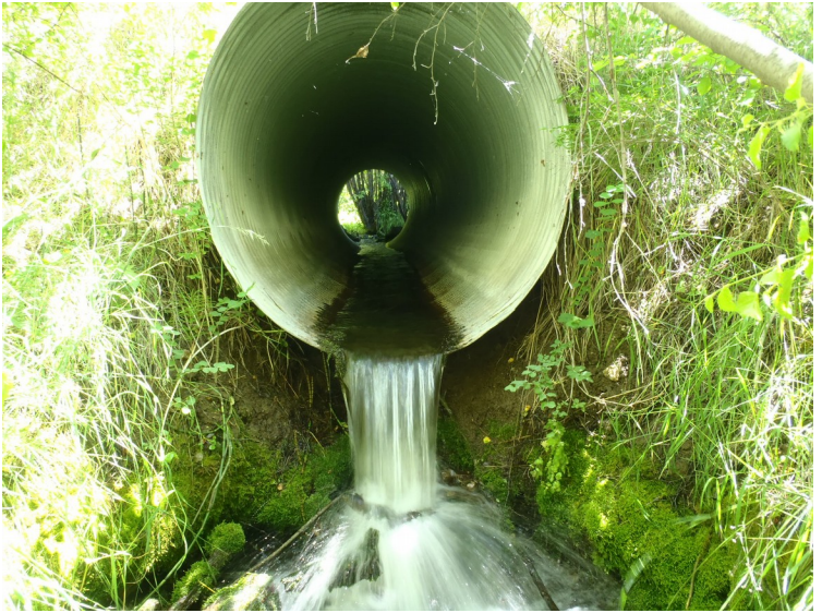
Buck Cr lower culvert outlet with no jump pool
