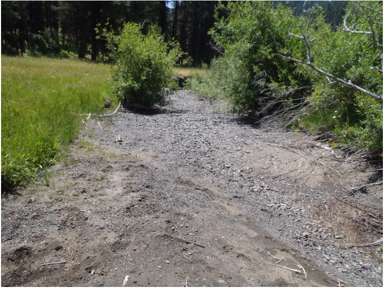
Channel showing silt deposits beginning to form
