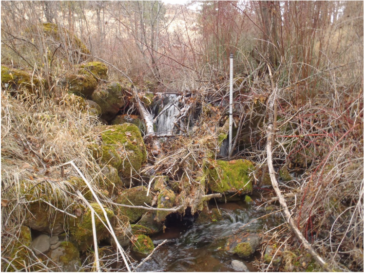
Falls pugged by debris with no jump pool available
