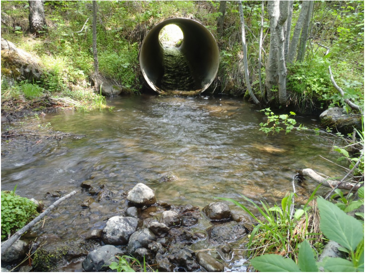
Thorn Cr culvert #1 has no perch and a good jump pool
