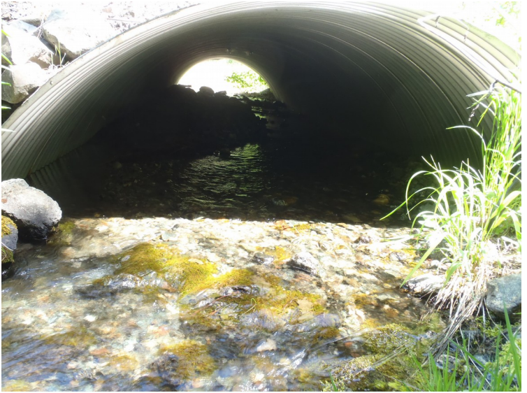
Outlet of culvert showing no perch and stream bed gravel through its entire length
