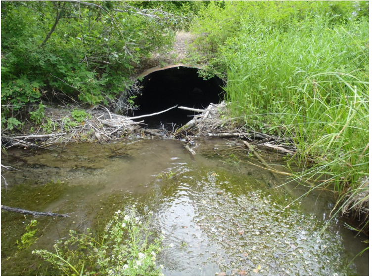
Culvert inlet with old beaver dam across it that could get worse
