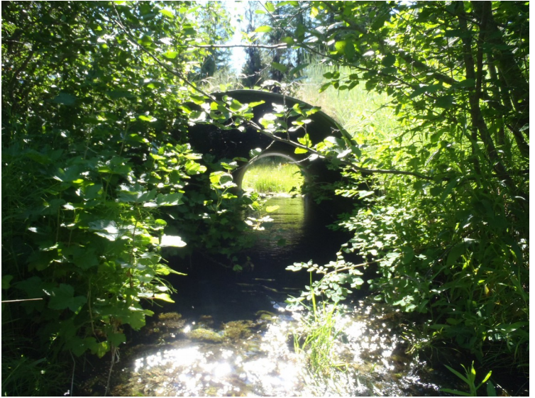
Culvert outlet showing no perch and stream bed material through its entire length
