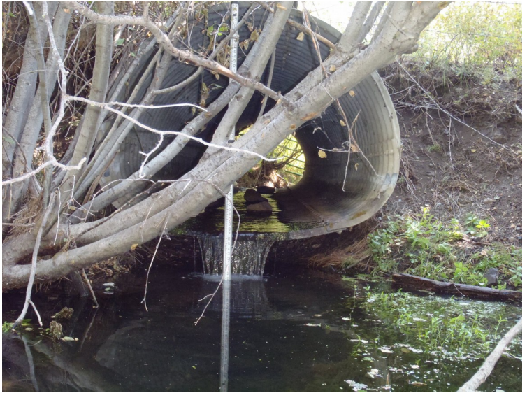
Culvert outlet showing flat slope with minimal jump height and deep jump pool
